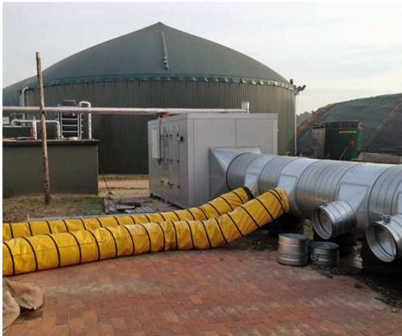
Heat Box with main ventilation channel
