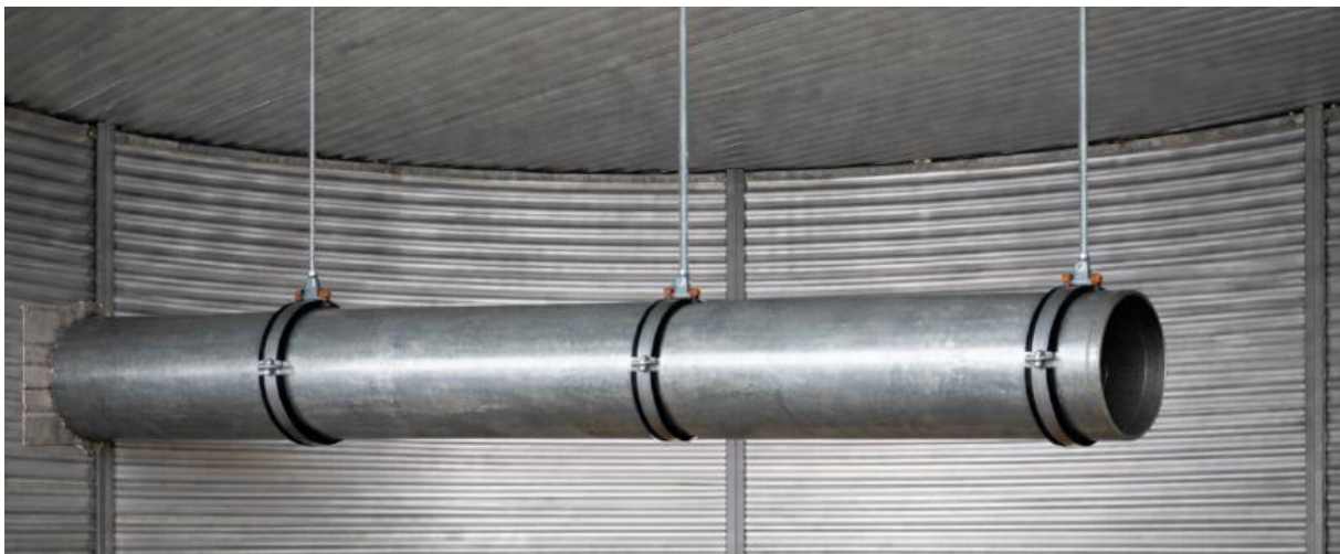
Figure 25: Exemplary pipe suspension of the ventilation line. It does not matter whether clamps with or without rubber inserts are used here.
