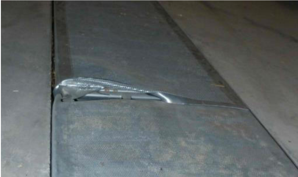
Figure 11: Damaged element due to incorrect layout of the covers.
