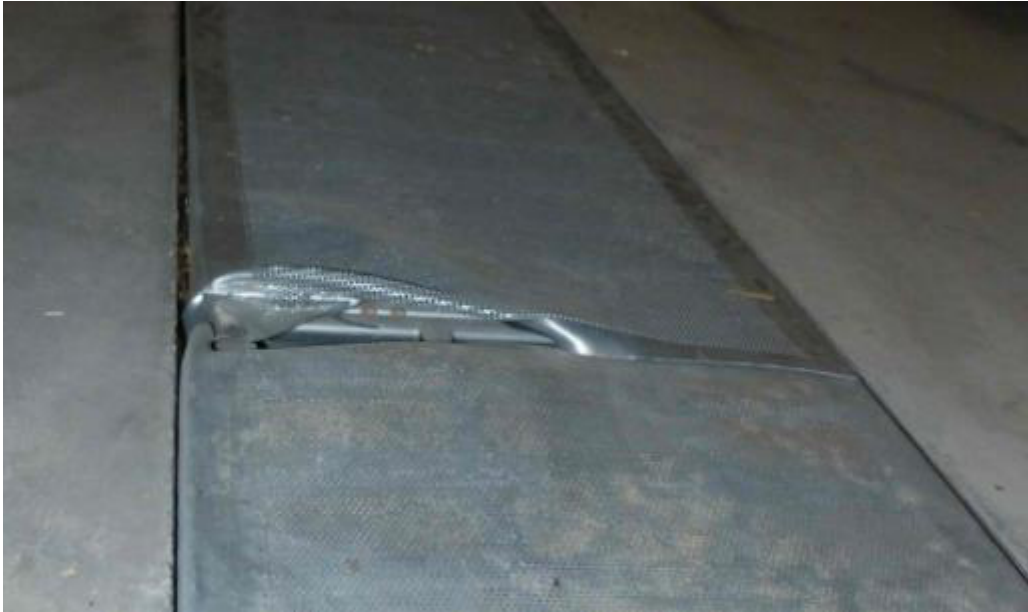
Figure 10: Damaged element due to incorrect layout of the covers.
